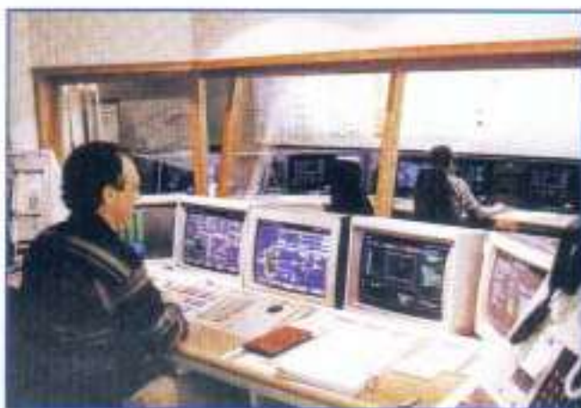
▲ Telecommunications & computer rooms
