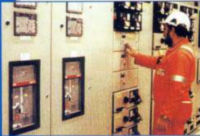
▲ Electrical switch gear rooms
