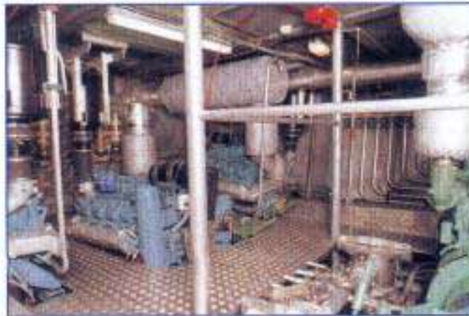
▲ Machinery spaces & cargo pump rooms on board marine vessels
