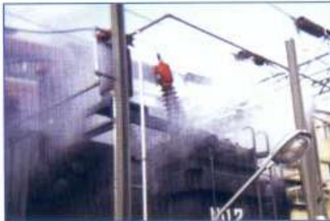
▲ Electric transformer sub-stations
