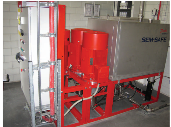
Compact SEM-SAFE® pump unit installed at Equinix AM3.
