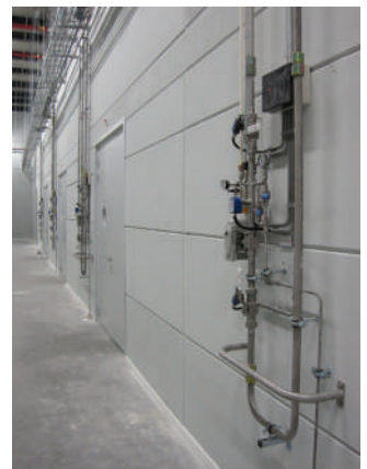
SEM-SAFE® pre-action section valve placement in Equinix AM3.
