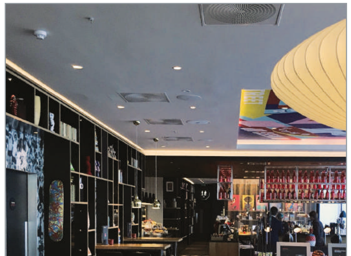
The SEM-SAFE® high-pressure water mist nozzles fits perfectly with the modern interior of CitizenM Shoreditch Hotel.
