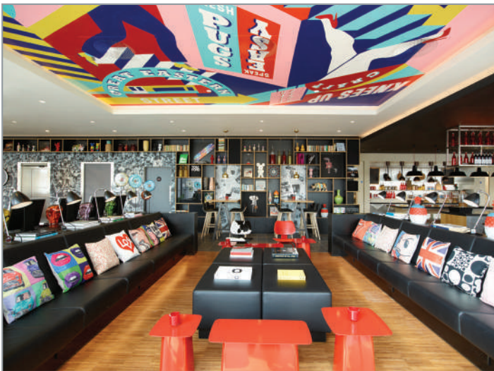
The dynamic and strikingly urban lobby area protected with SEM-SAFE® high-pressure water mist system from Danfoss.
