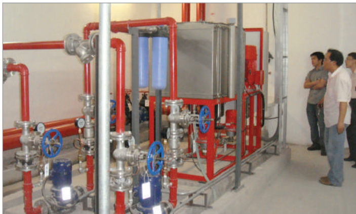
SEM-SAFE® pump unit installed in the project site.
